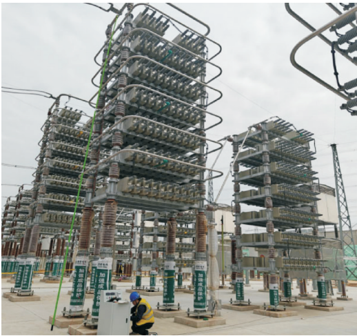
图8 换流站现场不平衡电流试验验证 Fig.8 On-site unbalanced current test verification for converter station
